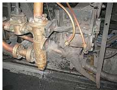
F09 - Class 15CA injector steaming along without an overflow pipe while Pat was busy sorting out a poorly fitting flange gasket.
