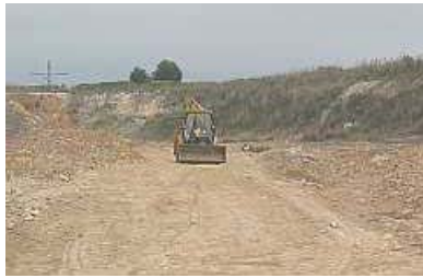
M01 🚛 Road clearing again. A Transnet front end loader is heading towards Knights Road as 🚛ve pulled over. The road is remarkably improved but we are looking forward to a tarred road by Shongololo Express.
