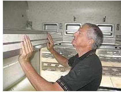
W03 ☹️ Wilhelm ☹️ Willie ☹️ Wehmeyer is inspecting an upper bunk in a 3 rd class compartment for cleanliness and damage in a Saturday of coach inspections. Lex and Willie are drawing up a list of both cosmetic and structural repairs that are required for our mainline coaches.
