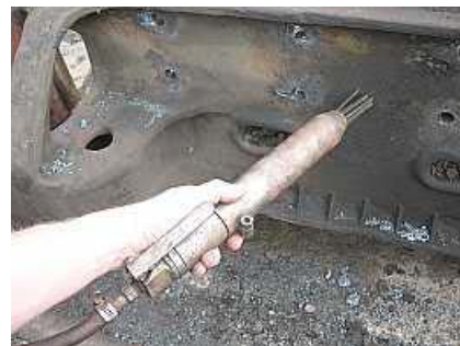
B03 ☞ A close up of the pneumatic descaling tool which Dawie and Shaun used in turn. (The vibration gets to be too much after a while.) Notice the metal shavings on the lower flange lip and the ground, the remnants of torched rivets.
