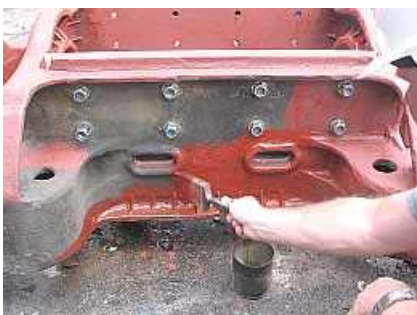
B13 Work threads converge. Piet Steenkamp sneaks in some extra primer paint around the newly fitted but still loose slide bearing nuts while the Bissel boys were looking for jacking components.
