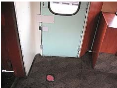
C01 - Completed sealed coach door with plating over the lock and latch cavities. You can see the grey coloured bolt plates a few inches above the floor. Now it just needs painting. Notice the rat treat in the vestibule.
