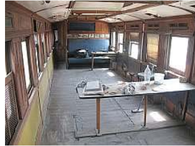
H03 Gutted coach interior after some cleaning. This used to be a sleeper coach. That blue seat at the end is one of the bunks against an intact compartment wall.
