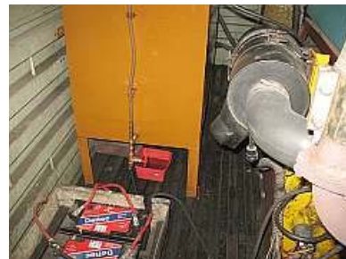
C03 - Relocated Generator Diesel Tank fuel intake. You can see the raised intake just above the lowest of the shut off valves. That red container under the tank marks where the original tap point was.
