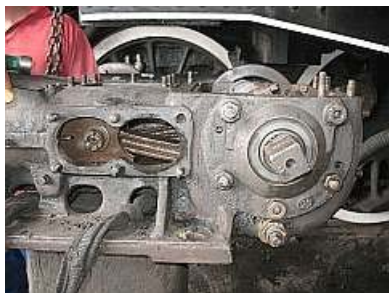
S04 Side view of the Stoker prior to crankshaft removal. Behind the inspection cover, you can see the LHS valve eccentric rod and the valve spindle's cross head.
