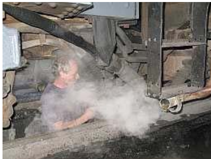
E22 Tight quarters. Andrew is just inserting the blanking disk into the locomotive side of the tender brake line. You can just see the disconnected tender brake line angling down in front of his forehead. The pipe in the foreground is the water feed for the RHS boiler injector.
