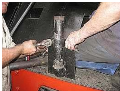
B10 The brake stand section of the pipe is clamped to the stand to provide something to work against. The dummy pipe has yet to be installed.
