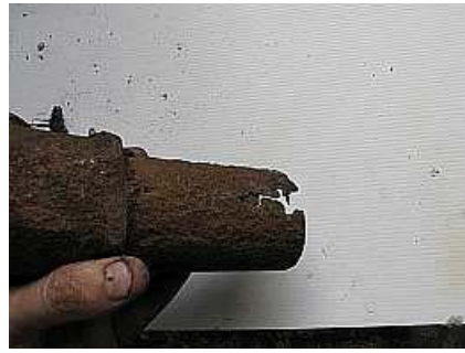
B03 Here's half the split in the very rusty dropper pipe.
