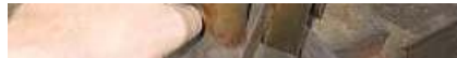
E17 A pair of castellated gland nuts halfway along the cast-iron shaft, which is visible spanning the two. These should be tightened by means of a c-spanner, not by a hammer and punch as we've so often seen evidence of being done.
