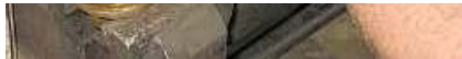
E16 Spinning in the nuts with a loose spanner, before laying it flat for the final tightening. The hex head for the pivot, visible just below the spanner, blocked access. The grid above the spanner is the air intake.
