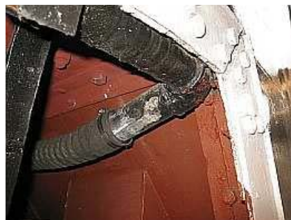
B12 The flexible pipe used to make the final connection to the angled train vacuum pipe. The front of the locomotive is to the right.
