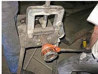
B05 A bit of grunt work cutting threads on a 2 inch pipe.
