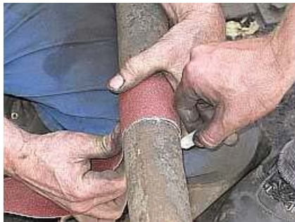
B04 Using a strip of sandpaper as a ruler, the edge of the pipe is marked off square around the entire circumference..
