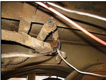
CW07 – Newly drawn incomer cable (White) protruding from the opened inspection elbow.
