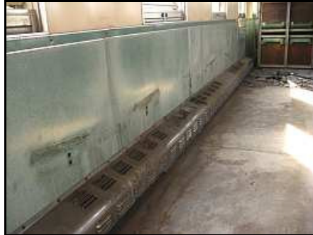
CW11 – Here's an original SAR spec coach heating system. These covers enclose a series of straight steam-filled heating pipes, with circular radiating fins. Heating steam used to come from the loco boiler and is the source of the photogenic steam leaks you see rising between coaches in movies. (Hogwarts Express, Polar Express, etc.) None of the steam heating systems are in current use.
