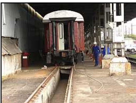
C01 – The first of the two full length white PVC conduits has been 'stuffed' with a pair of wires and the process of threading it under the coach has begun.
