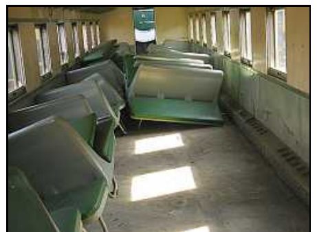
C09 – This typical 19mm marine ply coach floor has been stripped and cleaned. It needs to be power sanded before the new vinyl sheeting is laid. It is to be laid with Marley Tile Sheeting.
