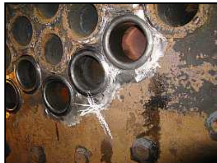
T09 – Two of three leaks at the firebox end. The cross marks the slightly weeping bead. That water is running from the tube at top right – a cracked existing bead.
