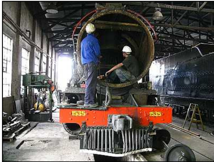
T00 – A chat and a review of the expected time of completion before the boiler could be pressurized. .
