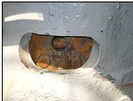
T02 – Oops. This washout plug on the right, opposite, corner of the wrapper plate had been left out. The draining water has slowed down to trickle. After leaking hoses and missing plugs, maybe we’d get it right on the third time.
