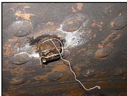
T10 – Putting the drip on things, the right front fusible plug is weeping through the threads. That tied on wire was for the inspection lamp.
