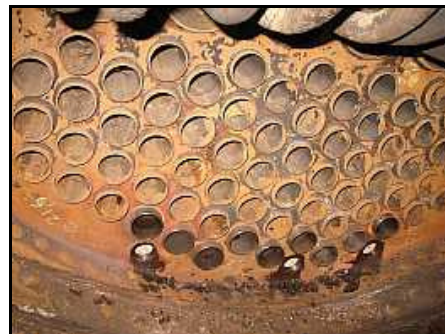
E06 – The three newly threaded washout plug holes still weeping oil from the thread cutting operation. The light brown colour visible through the holes is the rust-tinted lime scale that lines the boiler shell.
