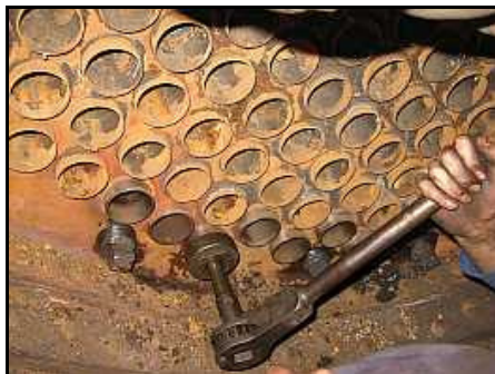
T08 – Putting the squeeze on the errant H 2 O, Dawie ratchets it up a few more turns. The dark coloured mess in the crevices is actually oil left over from when the washout plugs threads were re-tapped.
