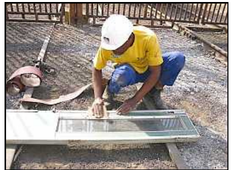
C06 – Spare gangway doors being cleaned for installation – here the oxidised and paint spattered aluminium window trim is being polished.
