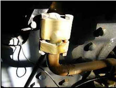
T04 – The right hand blow down is leaking a bit past the black rubber disk that was inserted to blank off the valve. The two through bolts were nipped up a bit and the leak promptly stopped.
