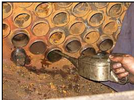
T07 – One of the first batch of seven tubes is weeping at the front tube plate next to the driver's side washout plug. Fresh MH Oil is being applied to the inner surfaces to lubricate the expander's rollers.
