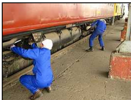
C02 – Miles (Left) feeds the new PVC conduit through the hangers for the coach's water tank as Coenie (Right) looks for the end.
