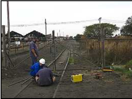
F01 – The gate gang working on the first set of gates to be installed today. This is the back entrance track alongside the western shunting yard. The vehicle road, also gated today, runs parallel to the right.
