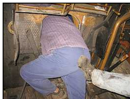
M03 * – Curious about the day's boiler tube beading work, a somewhat portly Mark Berry gets a little assistance to squeeze through the oval firebox portal on the Class 12AR. Said assistance was gleefully provided by Shaun 'Smudge' Ackerman.
