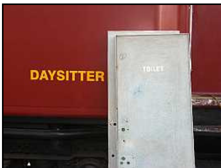
C07 – Removed and stripped toilet doors waiting for new white paint. All the hardware has been serviced and cleaned. These long-disused doors need to be rubbed down for spray painting but they are out of the way of the plumbing work.
