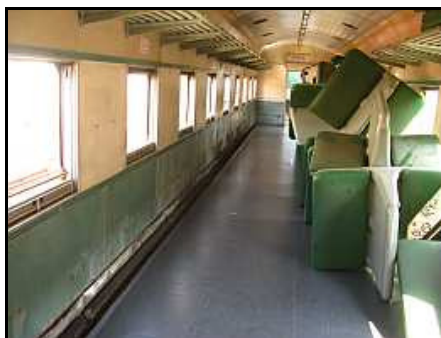
C17 – A newly laid vinyl floor in the currently unpainted coach No.25206. The seams are all heat closed and notice how the edges neatly wrap up into the open heater channels, The steam heating pipe is still in place in this photo
