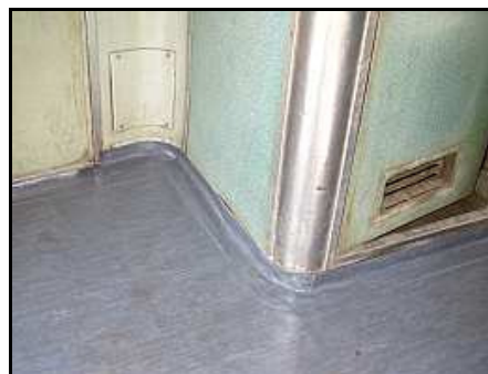
C18 – The free-form heat formed skirting wrapped around the circular section corners in the vestibule and forming a great water seal. The skirting on the green panel wasn't quite glued properly, but if Reefsteamers can fix locomotives, they can certainly glue a bit of vinyl flooring!
