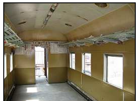
C12 – The two tone paint job for the walls. The entire ceiling is still to be painted white in this pic – but the curved quarter panels just above the luggage racks show just how dirty this coach's laminates actually were.
