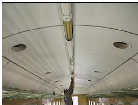
C16 – The painted ceiling having the converted 220V fluorescent lights re-fitted. Notice that the channels and support saddles for the lights and their lenses have been painted separately to match the ceiling.
