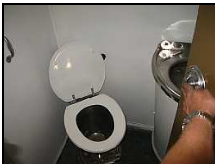
C08 – What a comparison! A gleaming white toilet compartment with a temporarily fitted and seated toilet. Luckily, the flooring in these compartments is still in good shape. (Because they were sealed up and out of use.)
