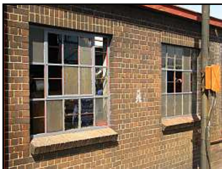
G01 – Three stages of work. The broken glass has been removed first and the empty frames are having new glass fitted. Then the existing, dirty glass will be removed, the glass cleaned and remounted in the frames with fresh putty.
