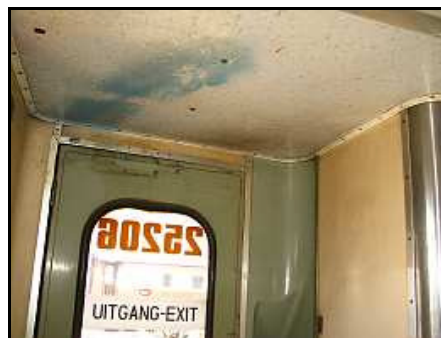
C09 – Grubby paint, yellowed laminates and a chemically stained ceiling. It looks as if the door closer had been 'repaired' and the hinges rubbed against the ceiling and someone used strong solvents to try to clean up, damaging the laminates.
