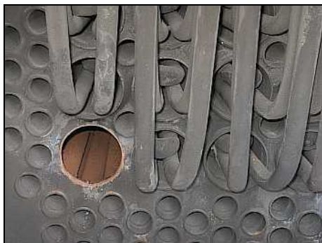
The known failed flue has been removed, leaving the characteristic ferrous-oxide coloured interior of the boiler exposed and providing a viewpoint for checking of adjacent flues. The difference between the smaller, empty boiler tubes and the larger flues, snugly inhabited by the super heater elements, is clearly seen.
