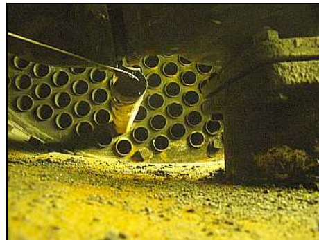
The boiler tube, which initially failed on a day-trip to Mariasburg, is blocked by the brake ejector exhaust while being withdrawn from the front tube plate. Upon closer inspection facilitated by the one tube being withdrawn – other boiler tubes were found to be wasted as well.
