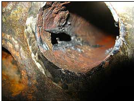
Here is a wasted boiler tube in the process of removal. The visible hole has just been cut by a torch to collapse the end of the tube to draw it out. However, the wasting and corrosion is clearly visible at the 10 – 11 o' clock position. Note the tube beading has already been ground off in this picture.
