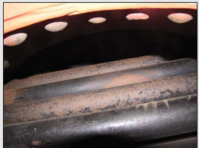
B06 – Boiler Tubes
